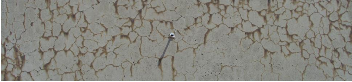
Figure 24. Example of ASR in the concrete
